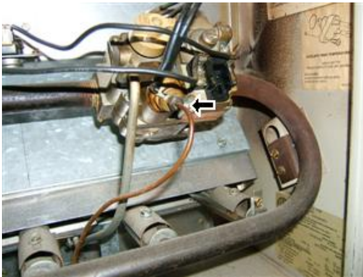
14.7 GAS PIPING Picture 1
