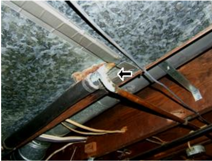
14.0 WATER PIPING Picture 1
