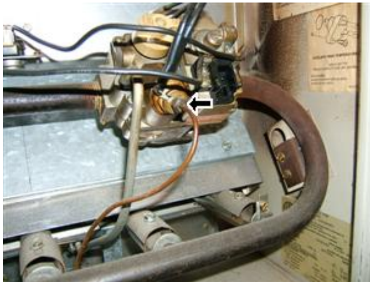
13.2 GAS / FUEL LINES AT UNIT Picture 1
