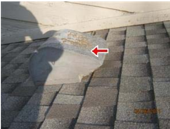
2.5 VENTILATION COVERS Picture 1
