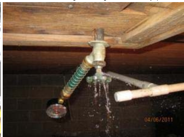
13.5 EXTERIOR FAUCET(S) Picture 1
