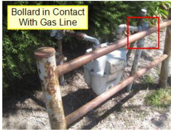
12.6 GAS PIPING Picture 1
