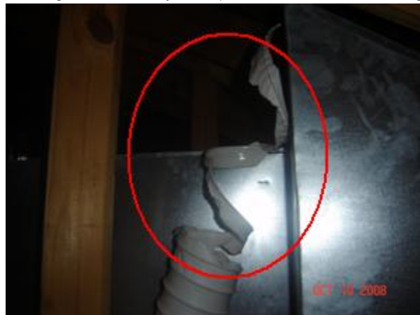
6.4.C VENTILATOR Picture 1
