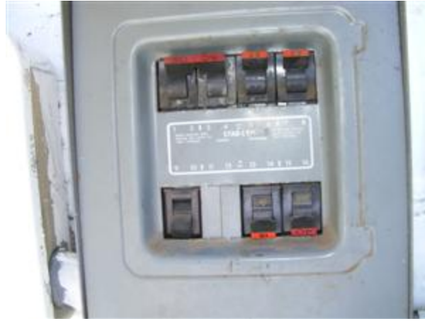
11.4 DISTRIBUTION PANEL Picture 1
