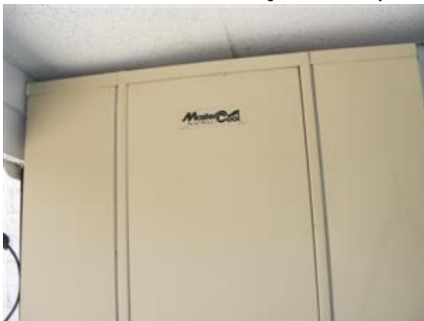
12.0 COOLING SYSTEM Picture 1
