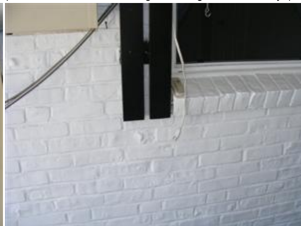
12.0 COOLING SYSTEM Picture 2
