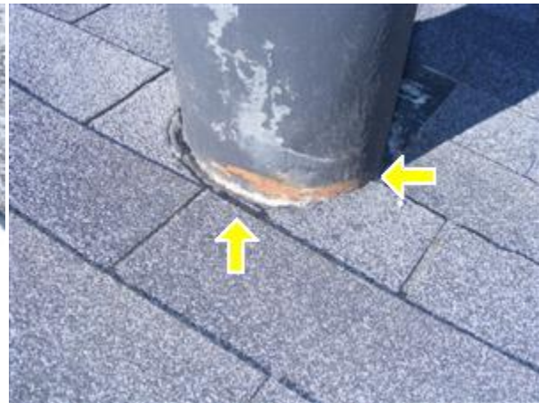
1.6 PLUMBING STACKS Picture 1
