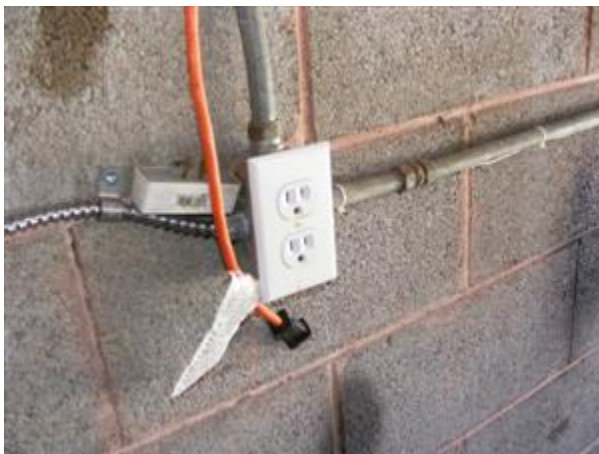
4.6 ELECTRIC / GFCI Picture 1
