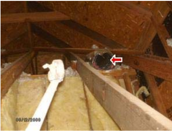
11.8 DISTRIBUTION SYSTEM Picture 1
