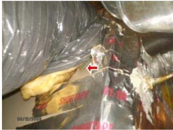
11.8 DISTRIBUTION SYSTEM Picture 2
